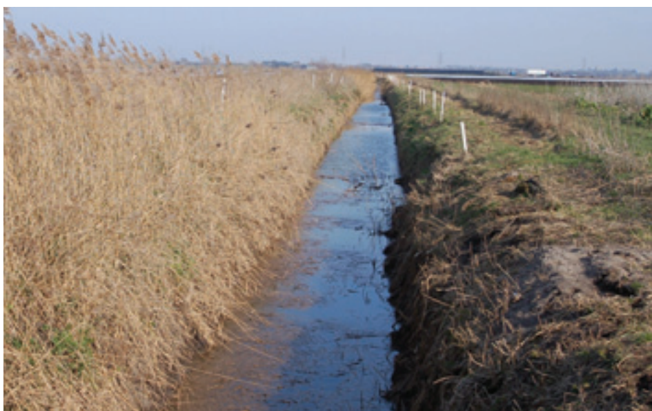
Ditch and dyke banks should be cut in alternate years, so that some well-grown habitat remains. Maintain shallow, sloping banks and avoid cutting ditch margins
